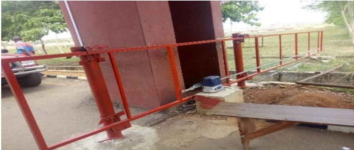
Figure 9: Installed and fully functional automatic gate
